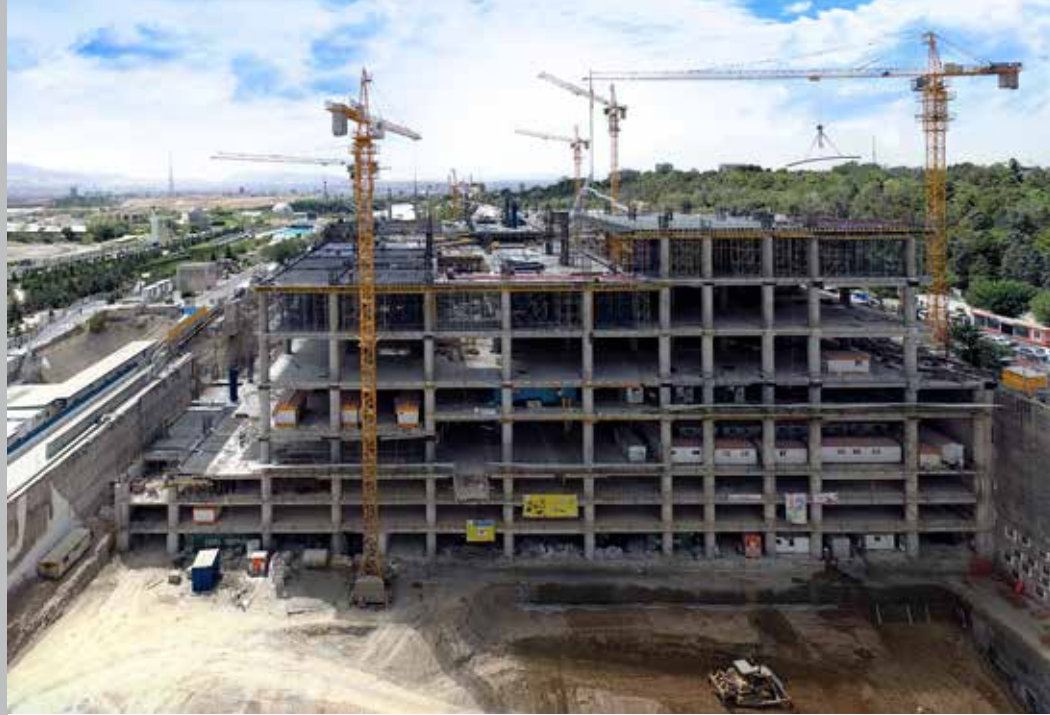
Atlas Plaza Commercial Complex Client: Setareh Atlas Pars Consultant: Heerim of South Korea Supervision Body: Pardisan Sazeh Consulting Engineers Type of contract: PC (Procurement & Construction) Location: Tehran, Iran Status: Completed
